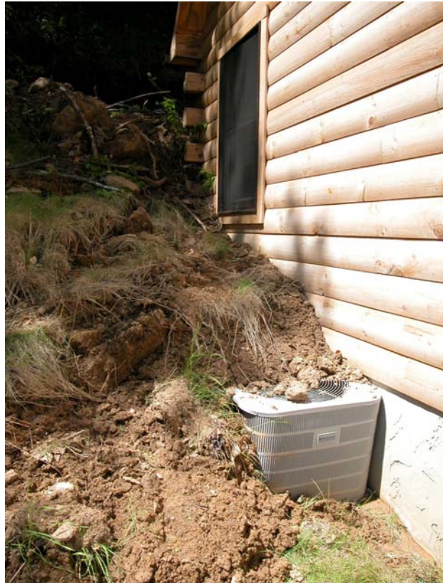
Lack of vegetated slopes or construction on too steep slopes can lead to slope failure
